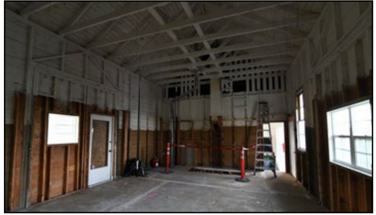
Interior walls removed from the east end storage side of the Depot, March 2021 Photo by Q Madp
